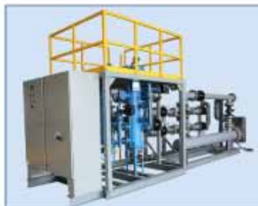
Filtration Process Skid
